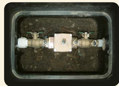
Double Check Valve Assembly on a domestic service line
