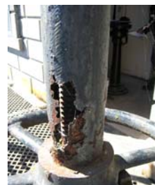
Wheeled gate operator stem cover, Outlet Gatehouse 6
