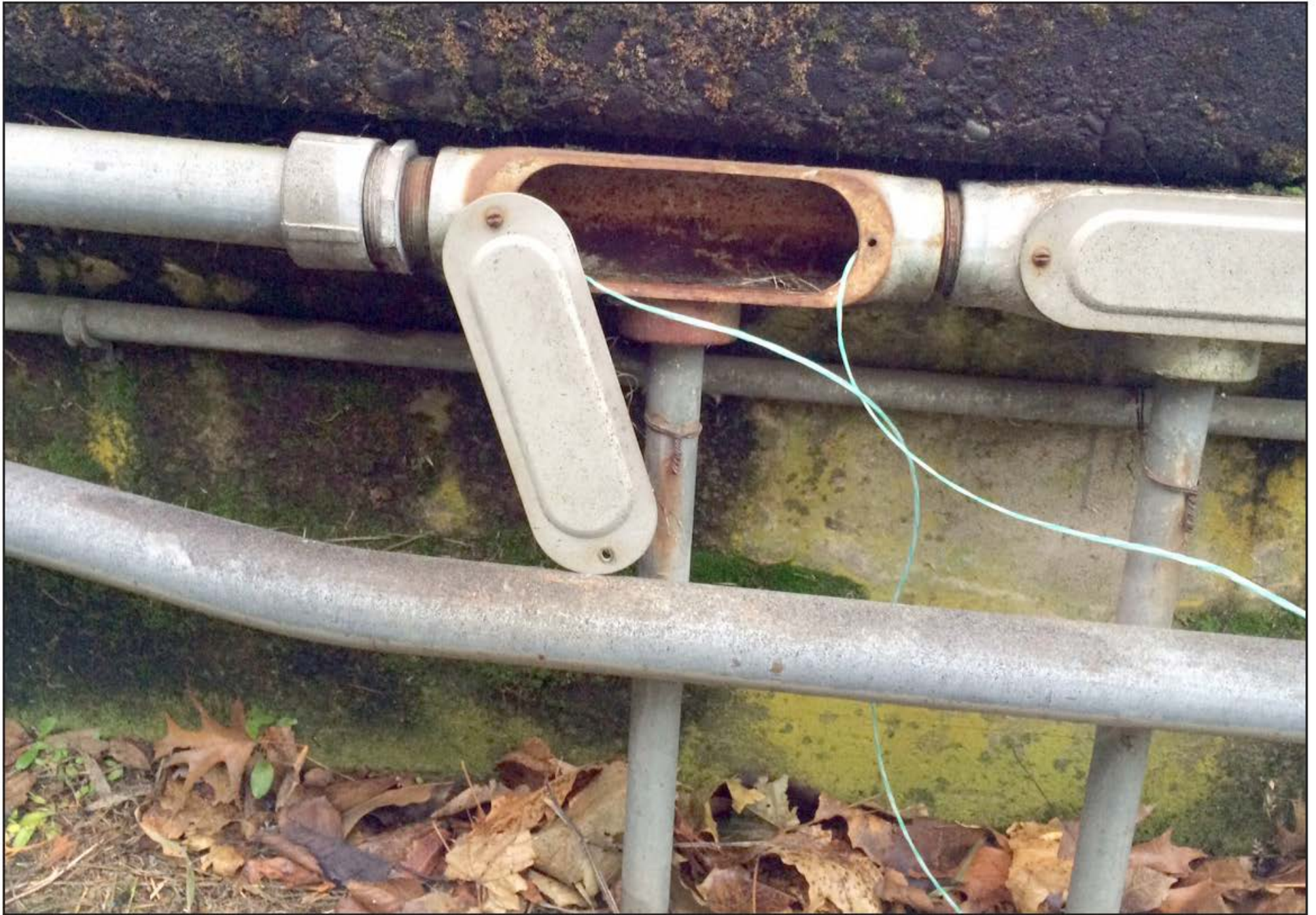
Non-historical electrical conduit has been thoughtlessly inserted, and then left unattended.
