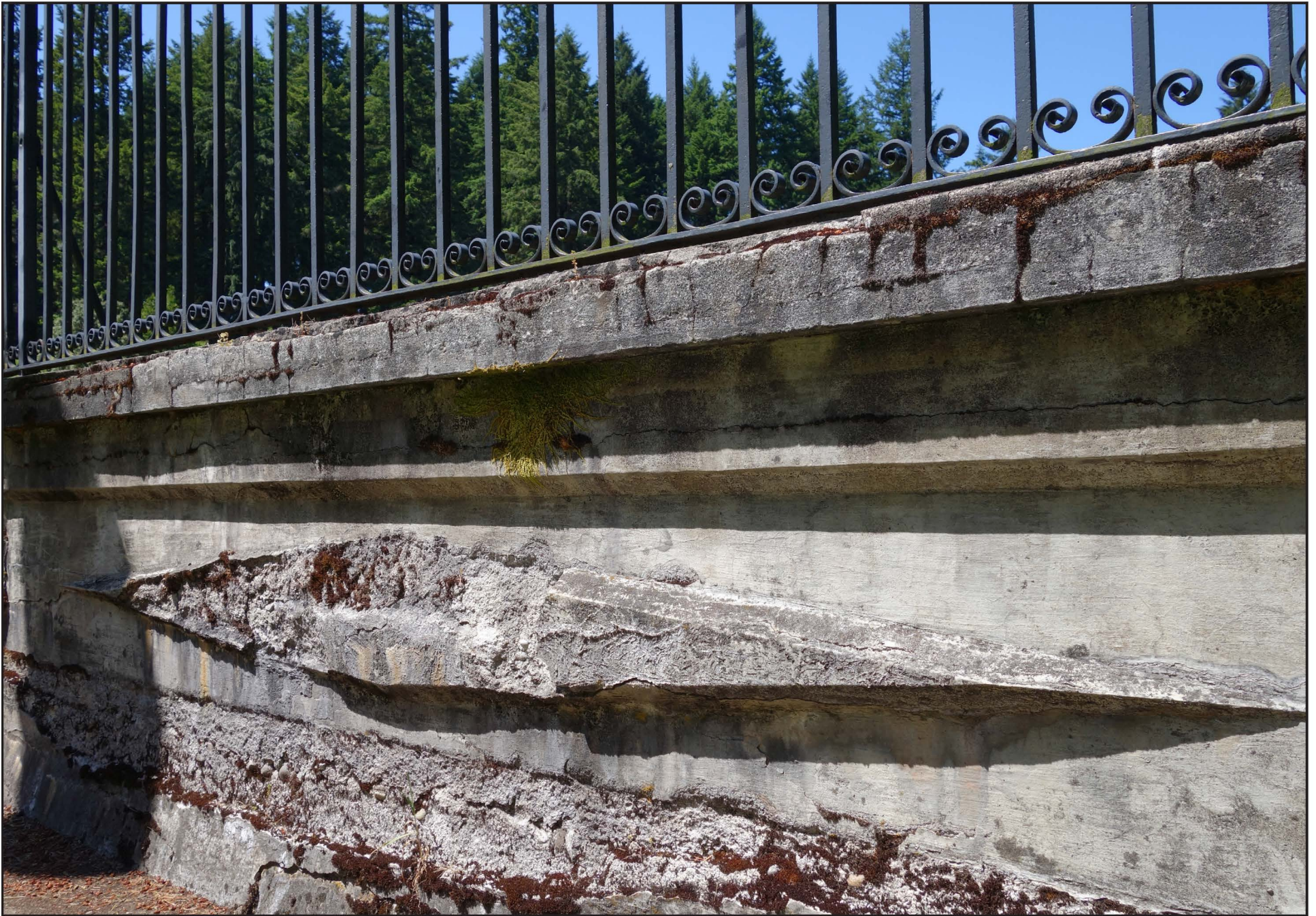
Carefully crafted decorative concrete designs are being allowed to crumble.
