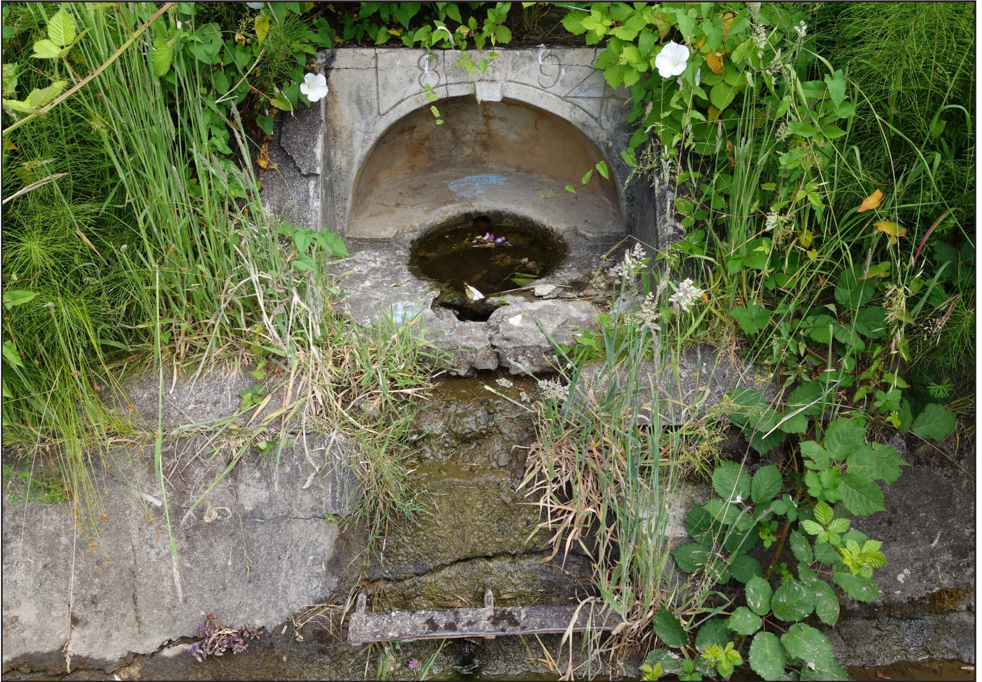
A unique and historically significant drinking fountain is lost in weeds and disrepair.
