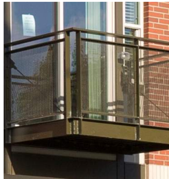
STEEL AND WOVEN WIRE MESH GUARDRAIL
