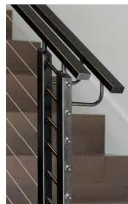
Painted steel rails w/ SST cables
