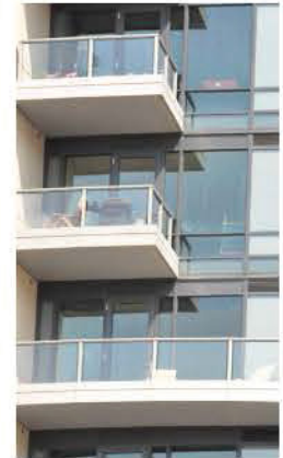
Glass and Pre- finished Alum Railing
