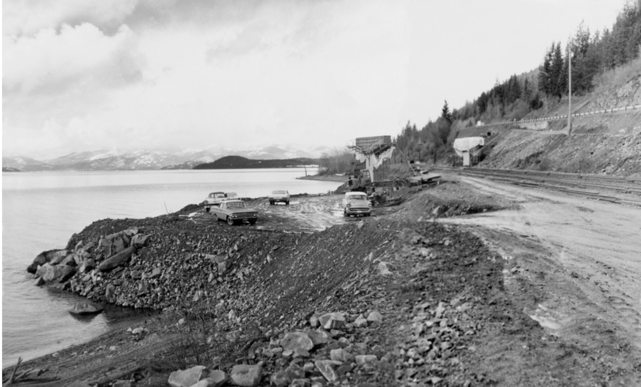
Figure 26. Lake Pend Oreille landslide. Hope Overpass site. Piers 2 and 3, on opposite sides of the Northern Pacific railroad tracks, are under construction in the background.
