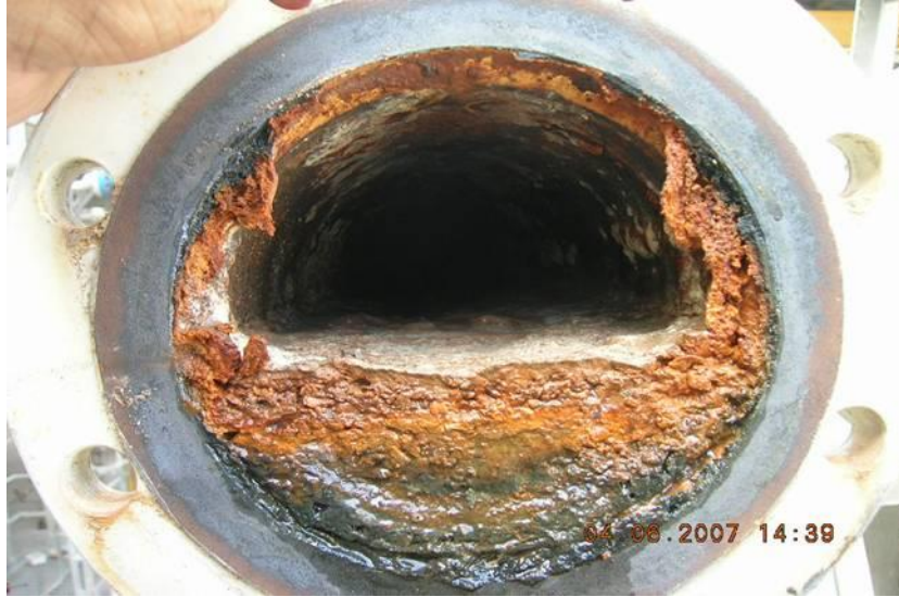
Neglected pipe. Portland Water Bureau maintenance management has been below industry standards for more than a decade. Biofilm slime can exert a great demand for chlorine which further puts water quality and public health at risk.
