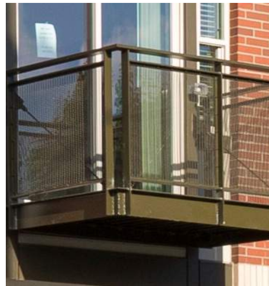
STEEL AND WOVEN WIRE MESH GUARDRAIL
