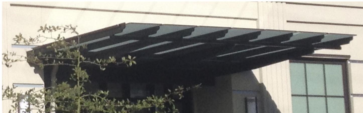
steel & glass canopy
