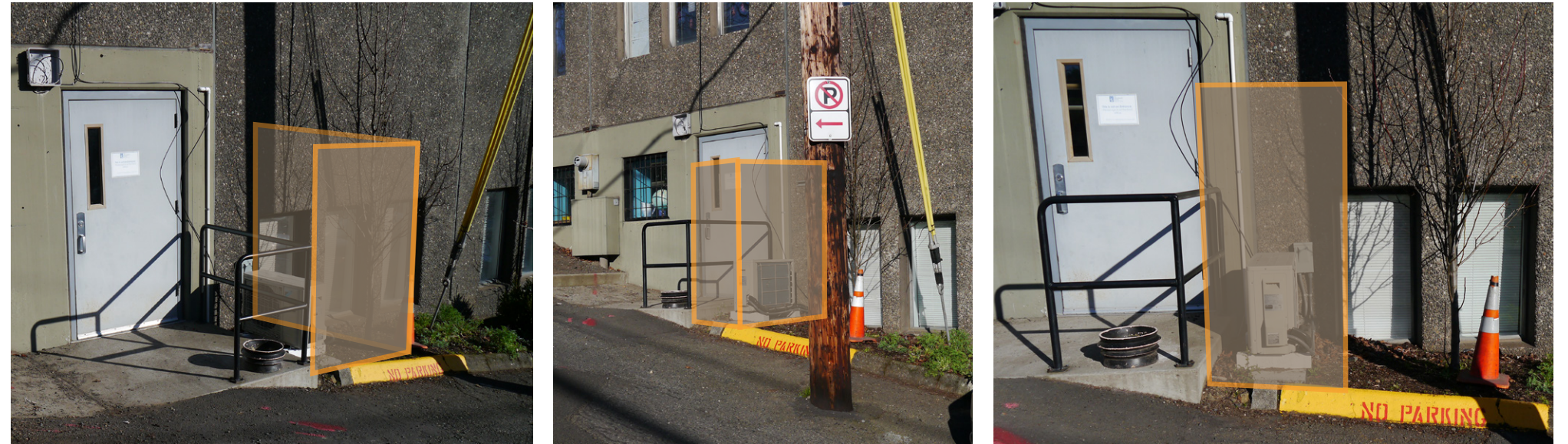
PHOTOS OF EXISTING GROUND-MOUNTED MECHANICAL EQUIPMENT AT HILLTOP BUILDING
