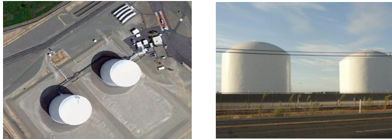
Figure 1: Suburban Propane’s two 12-million gallon double steel wall refrigerated propane tanks, separated from four 60,000 gallon pressurized tanks (LH picture, top right), by an earthen berm. Elk Grove, CA
