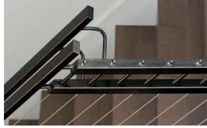
Painted steel rails w/ SST cables
