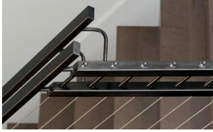
Painted steel rails w/ SST cables
