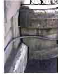
Joint to outlet house Reservoir 6
