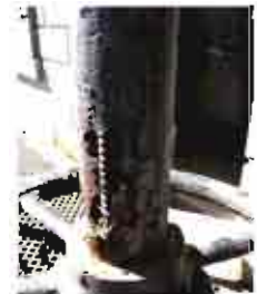
Wheeled gate operator stem cover, Outlet Gatehouse 6
