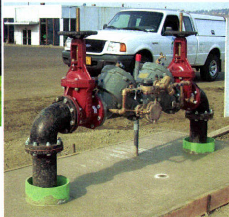
8-inch RP device in Portland
