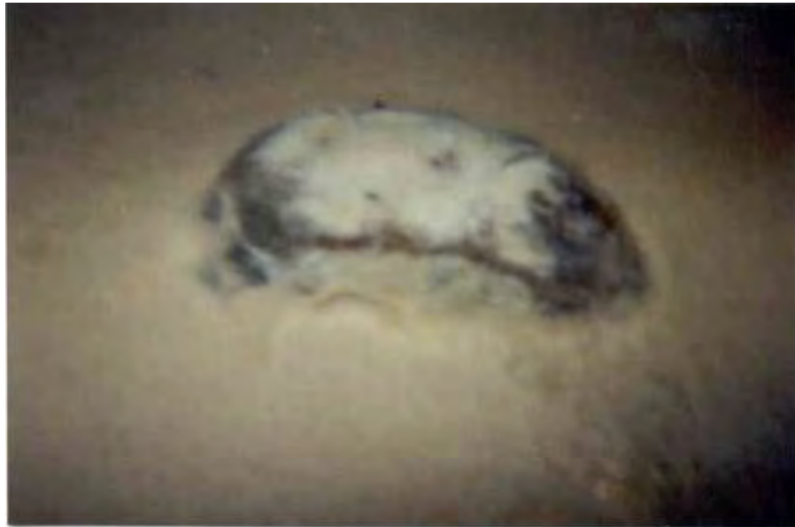
Deceased rat on layers of sediment in a covered reservoir. Common entry points for rodents, cats, and birds in covered reservoirs are hatch or access openings, vent pipes, structural cracks, and overflow pipes. (Ref. 58)
