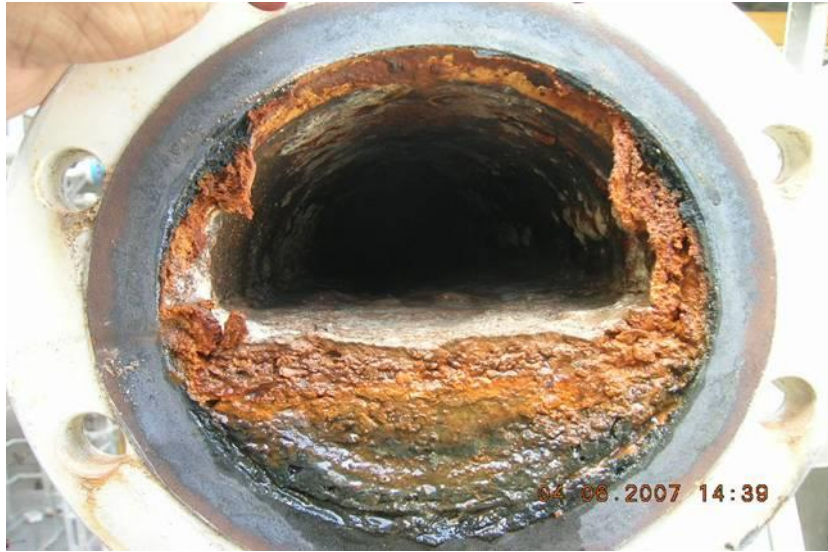
Neglected pipe. Portland Water Bureau maintenance management has been below industry standards for more than a decade. Biofilm slime can exert a great demand for chlorine which further puts water quality and public health at risk.
