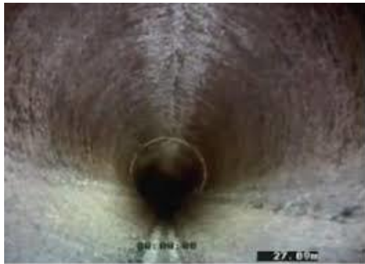
Scheduled routine flushing of system can remove microorganisms. Above is an example of properly maintained water pipe that has been routinely flushed.
