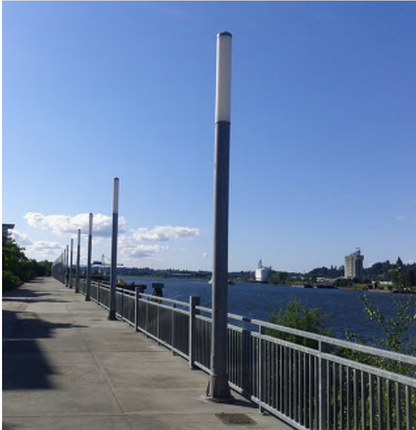
Greenway light fixture
