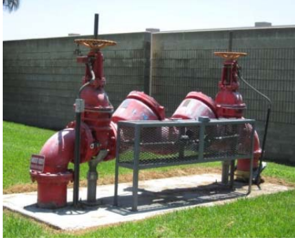
10-inch RP device in California
