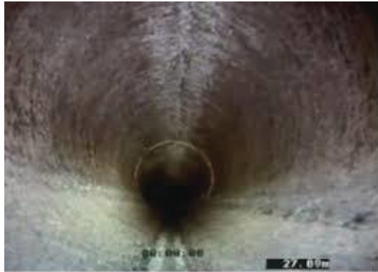
Scheduled routine flushing of system can remove microorganisms. Above is an example of properly maintained water pipe that has been routinely flushed.
