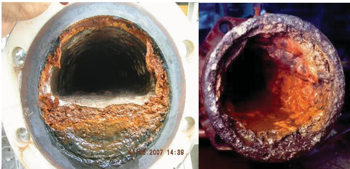
Example of water pipeline biofilm & sediment accumulation from years of Portland Water Bureau deferred maintenance and system neglect as source of alleged contamination resulting in “boil-water” notice on May 23, 2014
