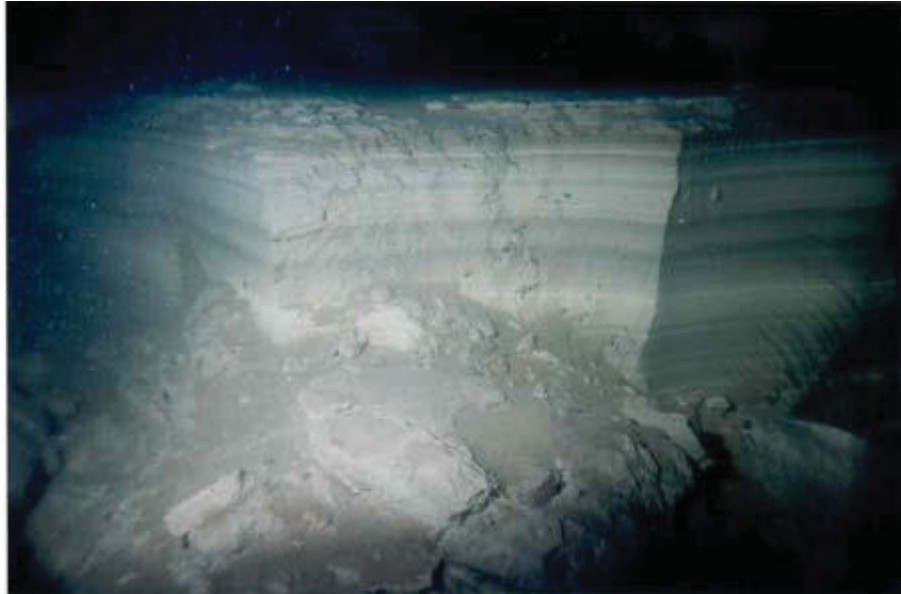
Unhealthy accumulation of post-filter media in drinking water: aluminum sulfate (alum) in seldom-cleaned covered reservoir. (Ref. 58)
