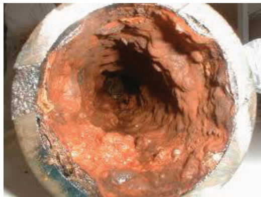
Appearance of biofilm buildup in water distribution pipes due to neglected flushing
