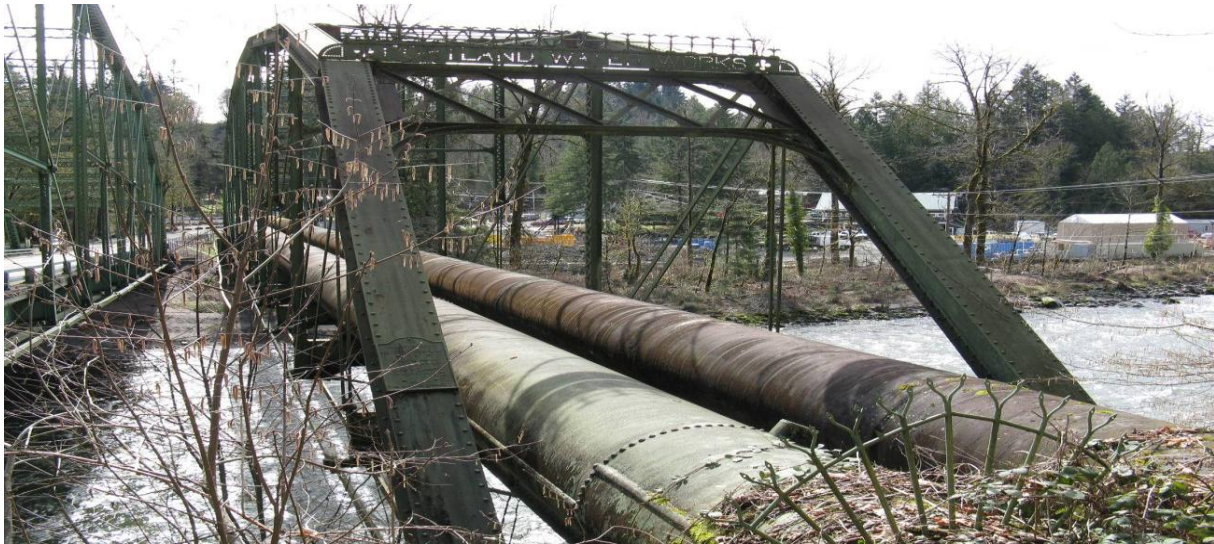
Figure 10. Two Conduits (2 and 4) crossing the Sandy River attached to a 115 year old Steel Truss Bridge.
