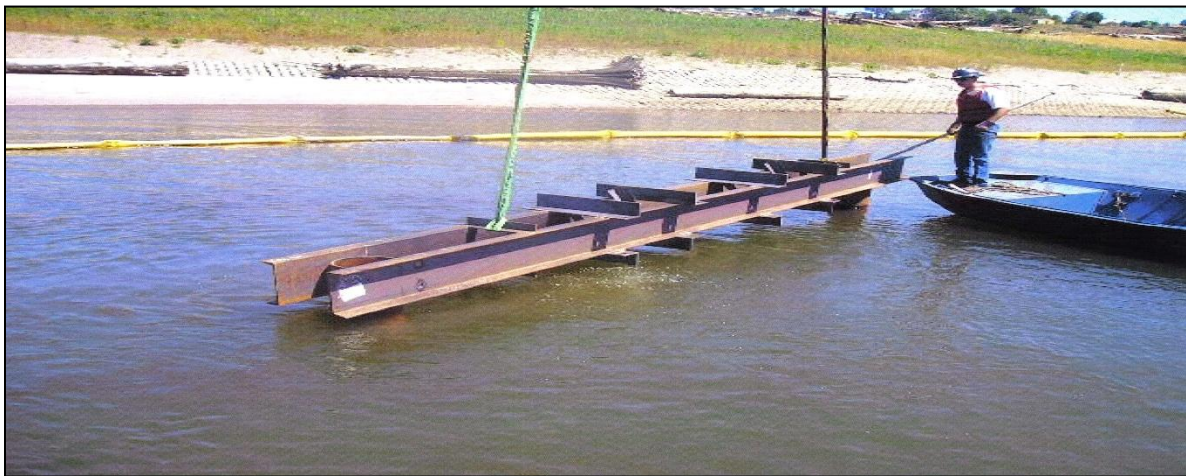
Figure 2. Construction and placement of the underwater pipe support assembly that was designed to support the weight of the pipes and the placement of the sediment cap (Guilds Lake/Willamette River Sanitary Sewer Pressure Line Repair Project)
