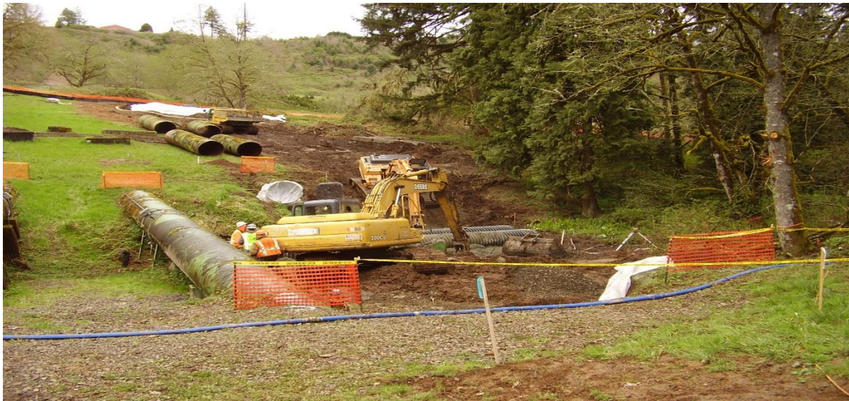
Figure 11. Burying exposed water pipes crossing drainage channels between the Bull Run and City of Portland.
