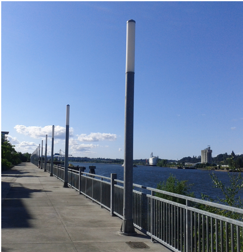
Greenway light fixture
