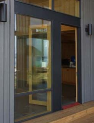
5 ALUMINUM CLAD WOOD WINDOWS AND DOORS
