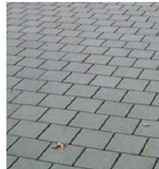
Mutual materials permeable Eco Pioria pavers- parking lot
