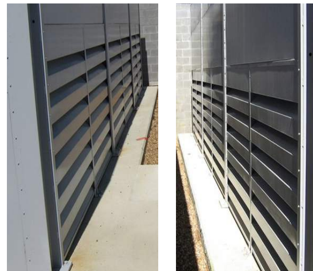
ACOUSTICS LOUVERS @ COOLING TOWERS
