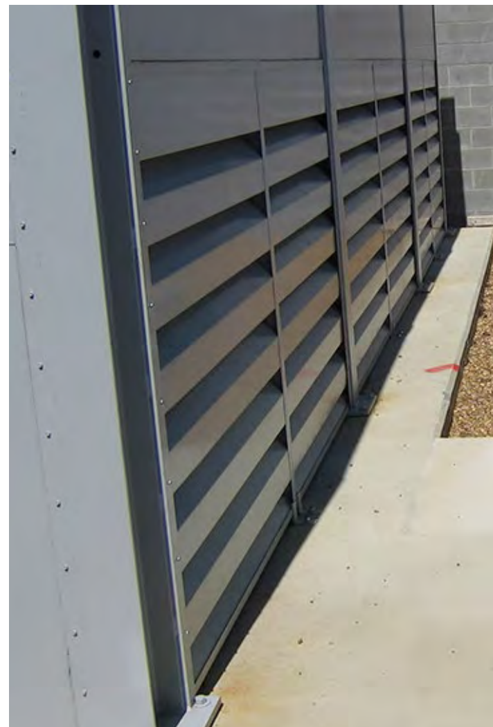
Acoustic Louvers at Cooling Towers
