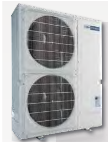
Split System Heat Pump - East Building
