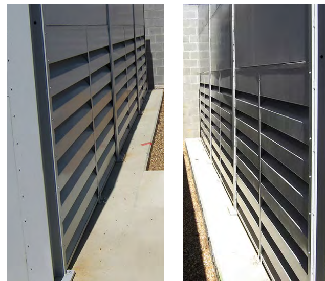
ACOUSTICS LOUVERS @ COOLING TOWERS
