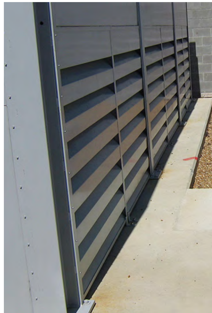
Acoustic Louvers at Cooling Towers
