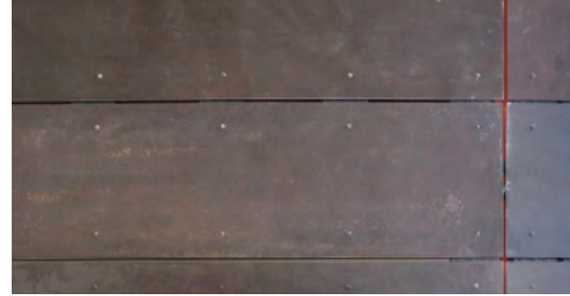
(05.45) LG Retail Entry & S. Micro Retail Steel Plate Panels w/ Exposed Fasteners
