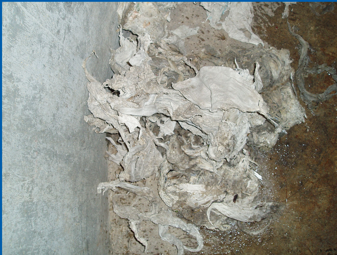
Rags Blocking Pump Station
