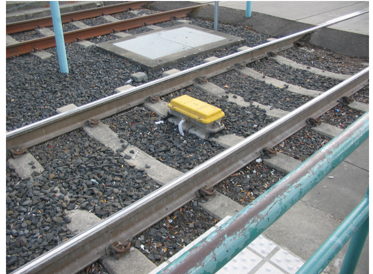
Automatic Train Stop Track Sensor
