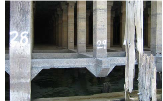
deteriorating wharf structure (photo: Flowing Solutions)
