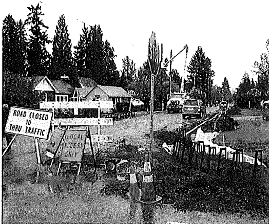
There was some project delay due to working during the rainy season.
