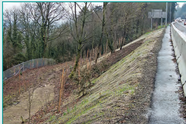
Erosion control measures on steep slope
