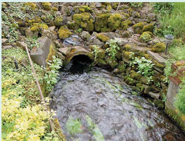
Before Crystal Springs Culvert Replacement – barrier to native fish passage.
