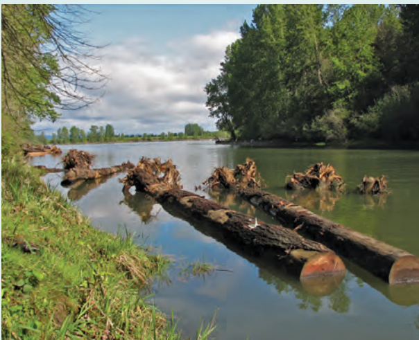
Installation of large wood at the Columbia Slough and Willamette River confluence project enhances critical habitat for migratory fish and wildlife.
