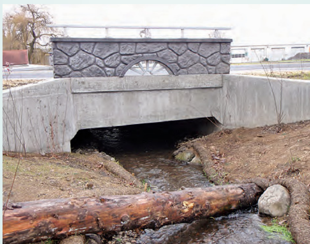
After Crystal Springs Culvert Replacement – native fish can migrate to spawning grounds.
