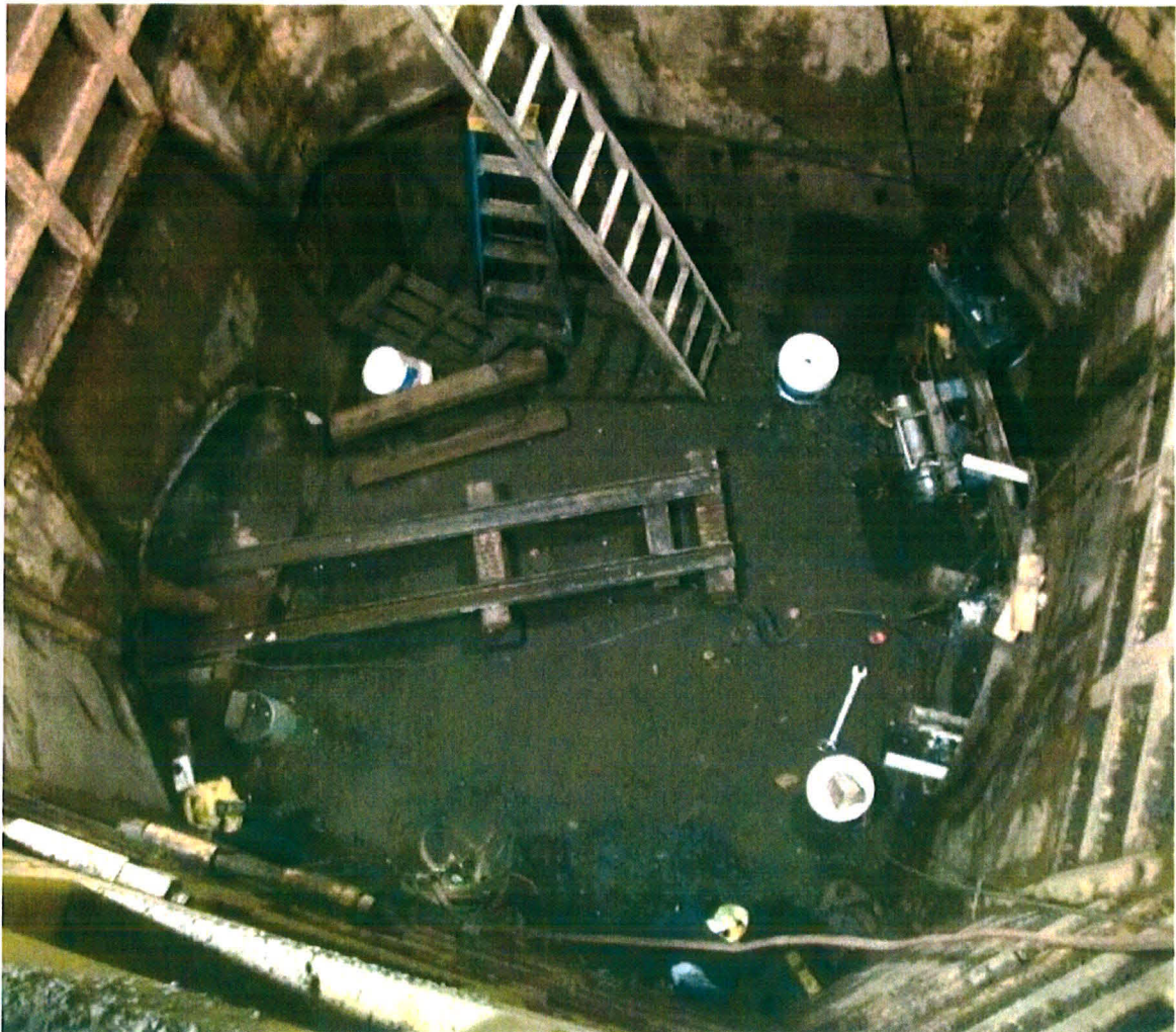
Rails being set for the 36-inch pipe to ride on to go into place
