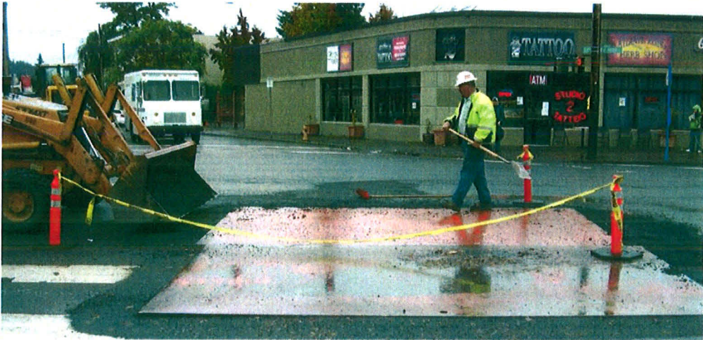
Sink hole covered with steel sheet.
