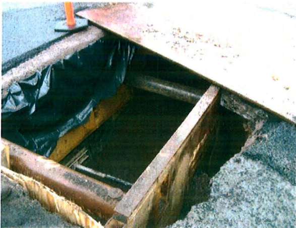
Sink hole due to bank failure.
