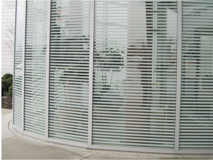
Dense stripes of internal frit on University Hospital's Twinsburg Health Center in Cleveland, by Westlake, Reed, Leskosky will overcome virtually all reflections. Photo: Christine Sheppard, ABC
