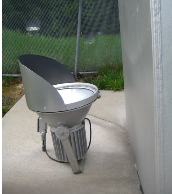
Floodlight at the base of the OHSU tram tower. Photo: Mary Coolidge
