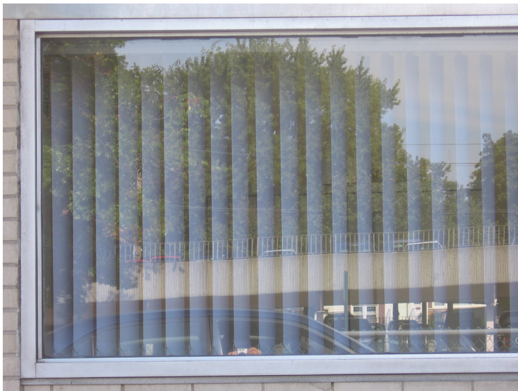
While patterns on the exterior surface of glass are most effective, blinds and curtains can help disrupt reflections. Partially open blinds, like those seen here, are most effective. Photo: Christine Sheppard, ABC
