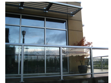
Transparent handrails are a dangerous trend for birds, especially when they are in front of vegetation. Photo: Mary Coolidge
