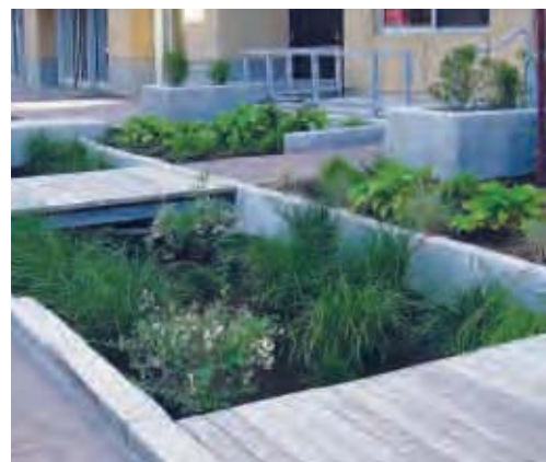
Vegetated filter box on SW Pennoyer Street
