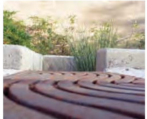
Vegetated filter box at SW 12th and Montgomery
