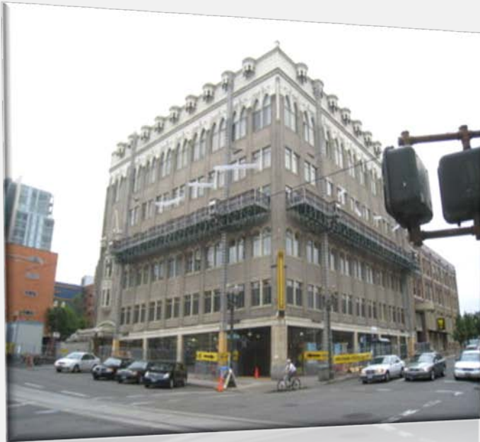
Chaucer Court provides 83 units of affordable rental housing for the elderly.
