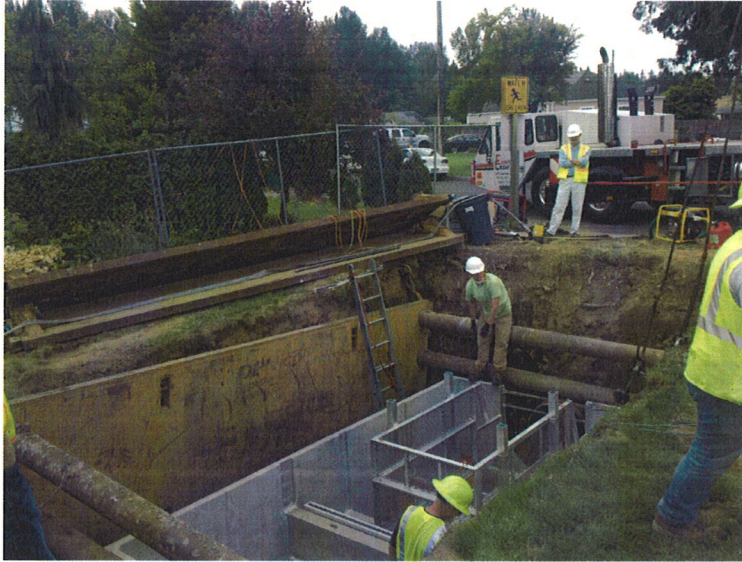
Installing Pollution Control Vault called a Bio Clean NSBB (nutrient separating baffle box)/Water Polisher. The purpose of the Vault is the processing of storm water with controlled upstream surcharging and targeting removal of bacteria, mercury, other metals, total suspended solids, oxygen-demanding substances, nutrients, oils and grease including various hydrocarbons, and bacteria, trash and debris prior to discharging downstream to the Columbia River.
