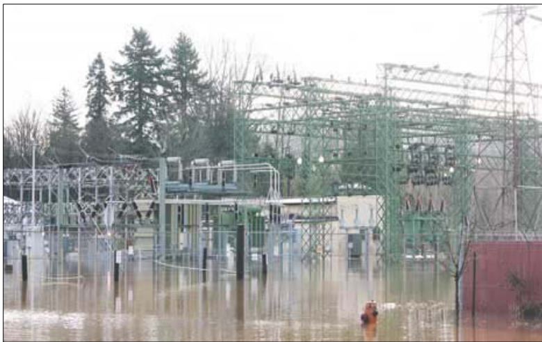
Foster Substation, 1996 flood
