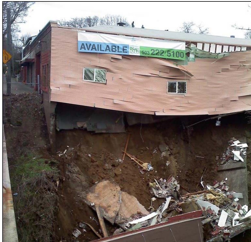
Landslide on NE 21 st , 2009
