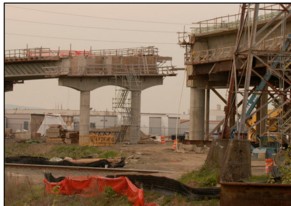
Funding for critical transportation projects like the Lombard overcrossing is needed to maintain the health of our industrial districts. (photo credit: Port of Portland)
