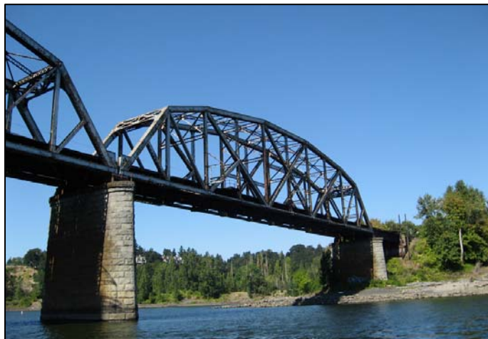
The BNS&F Railroad Bridge offers a potential rail with trail linking Portland's east and west sides for both commuting and recreational pursuits.
