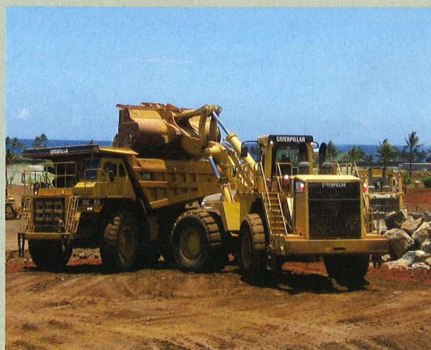
Large rock that will later be used as jetty stone at the Kikiaola small boat harbor is loaded into a 777 haul truck as part of a mass grading project supporting the construction of the first seven holes of an 18-hole golf course in Koloa, Kauai.
