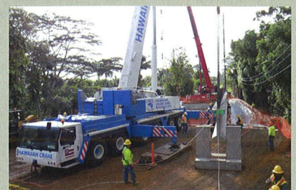
Skillfully choreographed crane picks eased the process of placing the six, 110-foot precast concrete girders for the Kilauea Stream Bridge.
