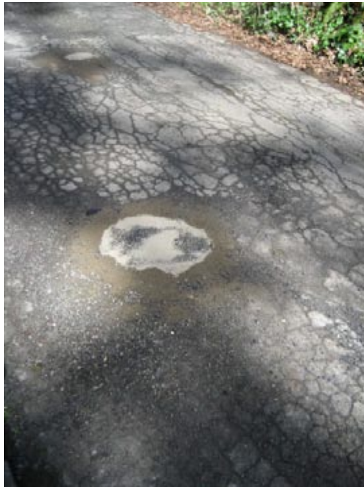
Figure A-3 Pothole filled in deteriorated street
