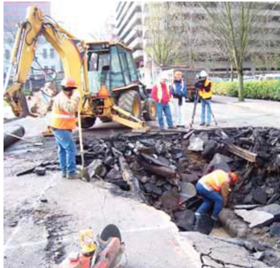
Figure 12 Water main break
