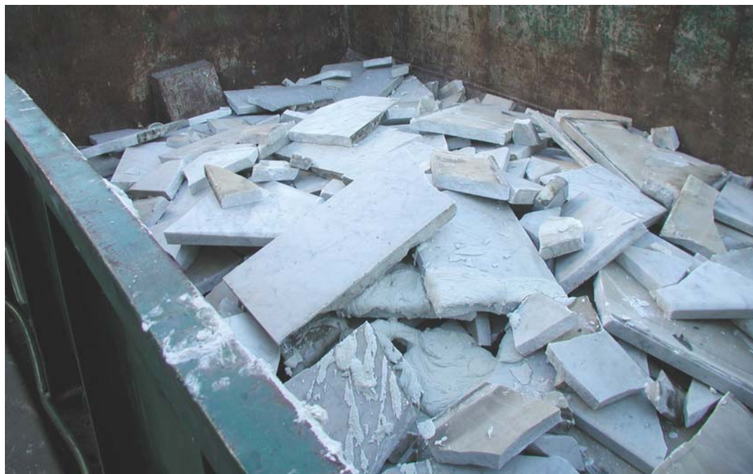
Drop box container outside of City Hall with pieces of the removed marble stairs
