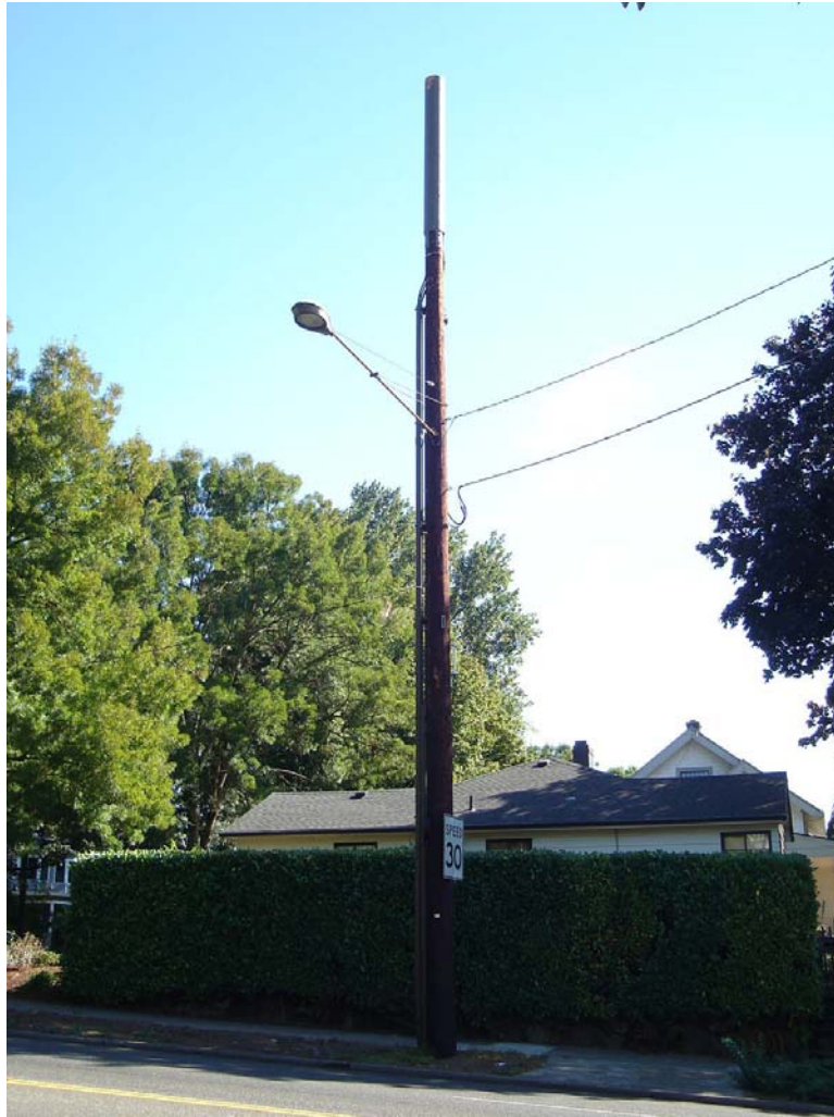
Canister antennae on replacement pole NE 39 th & Burnside
