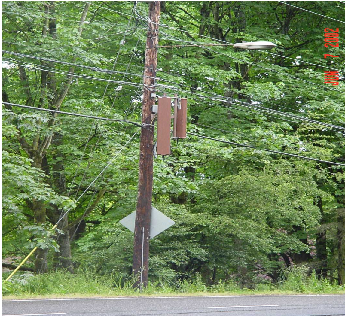
Antennae on existing pole on West Burnside
