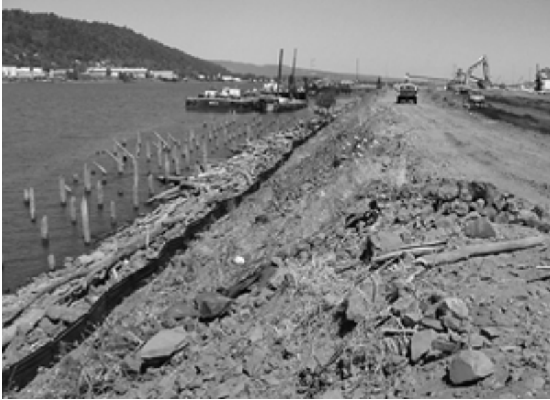
Before bank stabilization at Terminal 4
