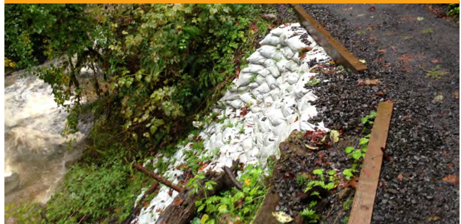
Lower Macleay Trail was damaged by a landslide.
