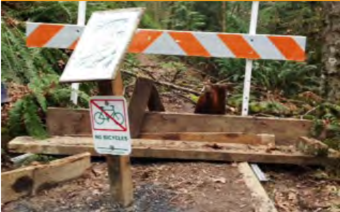
This bridge collapsed in 2012, closing part of the Maple Trail loop.
