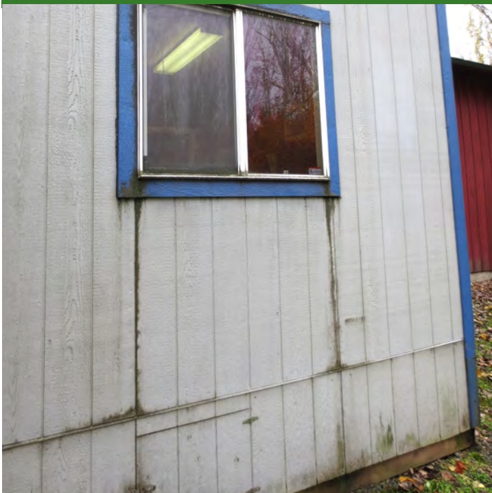
The trailer office at the Urban Forestry site is leaking and past its useful life.
