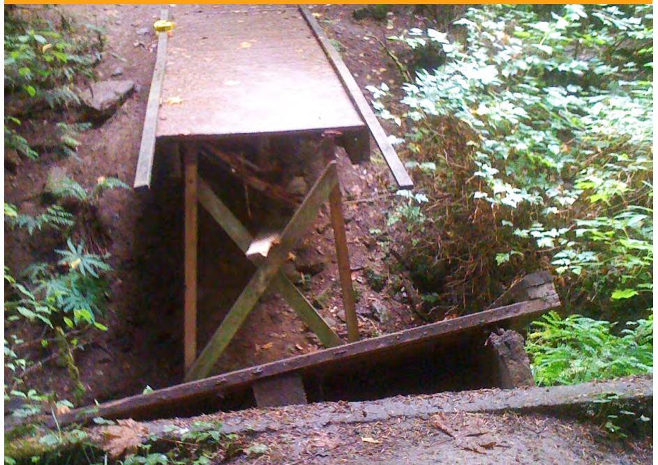
This bridge collapsed in 2012, closing part of Forest Park's Maple Trail.
