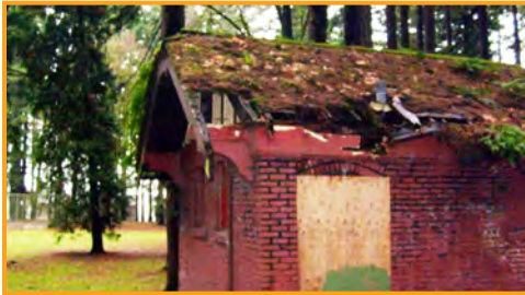
This restroom in North Portland's Pier Park is not ADA accessible, and has a severely damaged roof.
