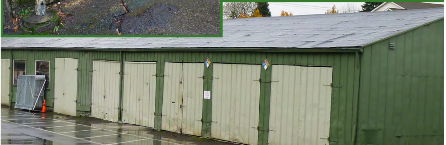
This building at Mt Tabor Maintenance Yard is held together by steel cables to prevent collapse. It is beyond its useful life span.
