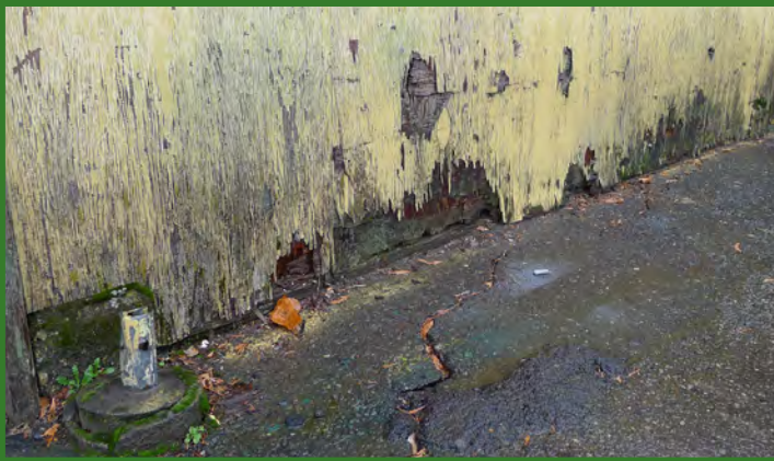
Structures at Mt Tabor Yard are beyond cost-effective repair.
