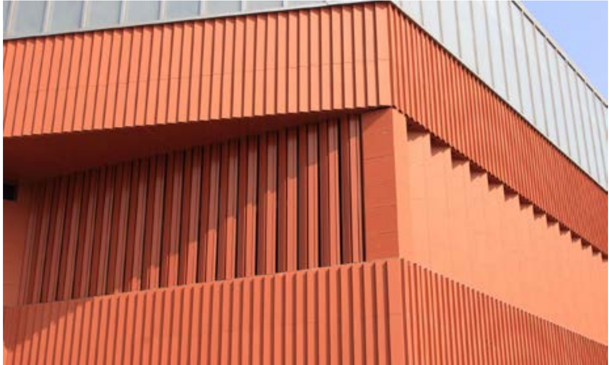
TERRACOTTA TILE RAIN SCREEN
