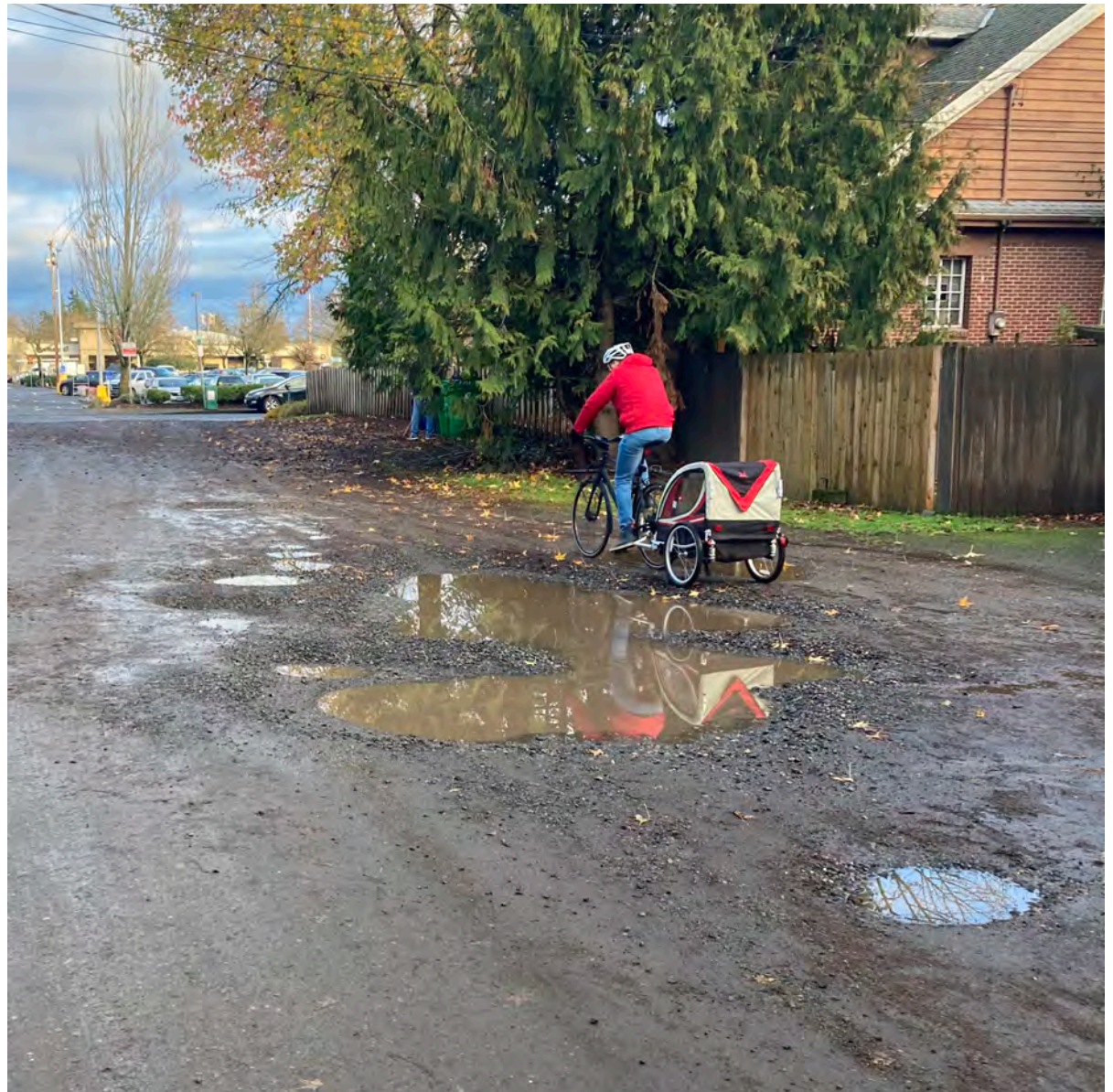
A cyclist navigates around water-filled potholes on an unpaved street in the Woodstock Neighborhood
