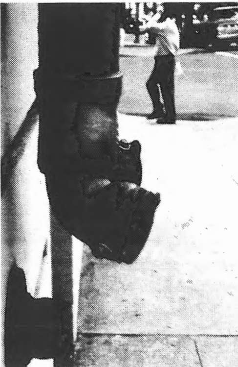
Elements such as standpipe systems may project into the Frontage Zone. Care must be taken to assure compliance with the ADA.
