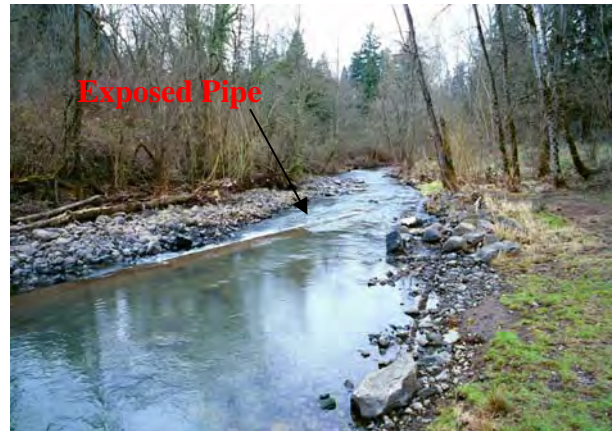
Photo 2a: Exposed sewer pipe crossing Johnson Creek at Tideman Johnson Park before restoration.
