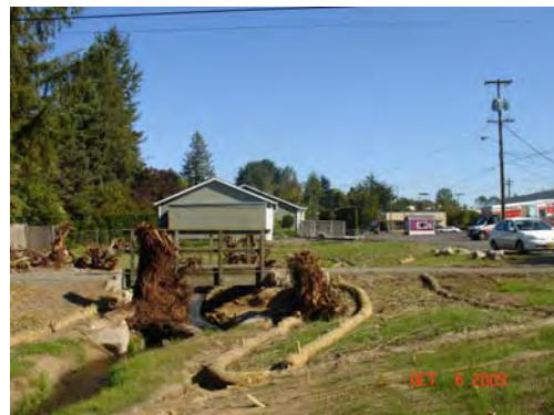
Photo 9b: Errol Creek post-construction. Vacating SE 44 th Ave allowed Errol Creek to be daylighted and fish passage to be restored.
