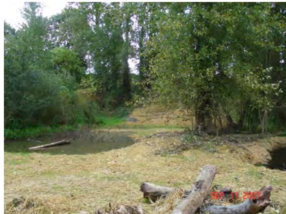
Photo 13a: Errol Wetlands in 2007, post construction, prior to revegetation. Ponds are clearly visible.
