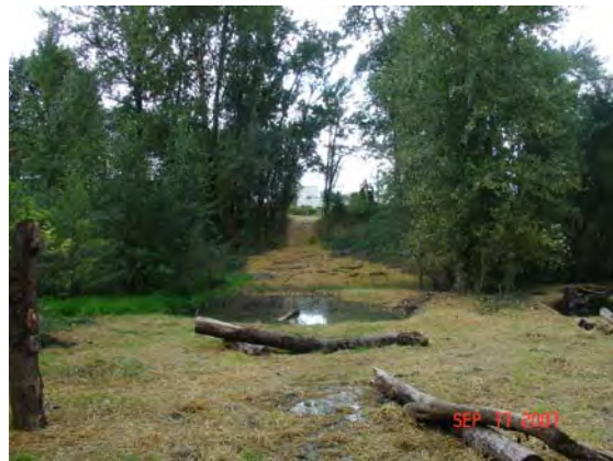
Photo 12b: Errol Wetlands post-construction, culvert is removed and multiple ponds are created in the wetland.
