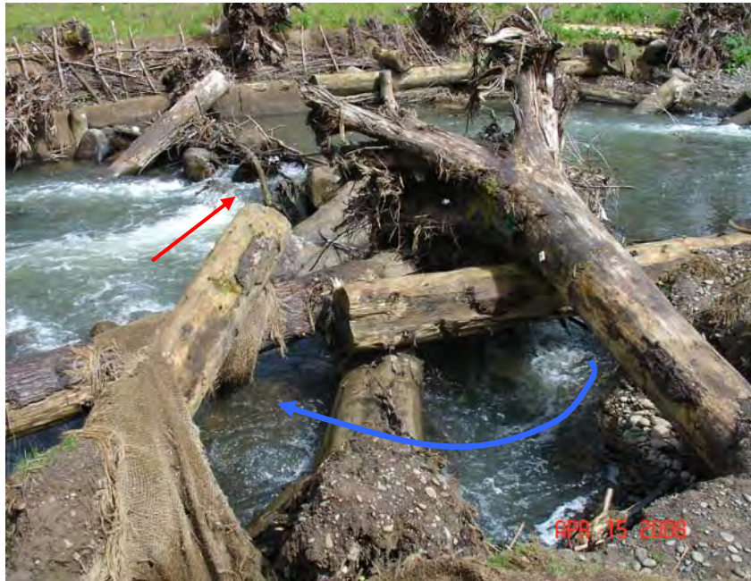
Photo 4: The lower most engineered logjam at the Tideman Johnson Restoration site. The red arrow shows the center of the stream which is being blocked by debris. The increase in resistance diverted stream-flow, causing bank erosion and exposing buried logs (blue arrow).
