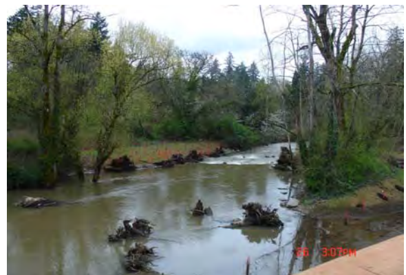
Photo 2b: Tideman Johnson Park post-restoration project. Pipe is re-buried, overflow channels were created, and large wood was placed in the channel.
