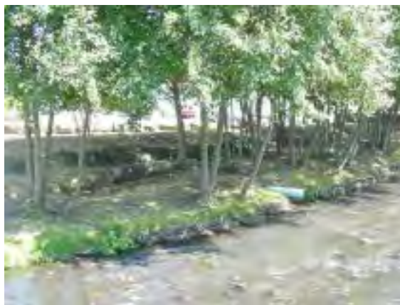
Photo 1-4: Looking east from west bank of Johnson Creek. This stand of native red alders should be preserved and the native vegetation enhanced to improve the riparian corridor along this section of the creek. Outfall pipes, such as the one shown here, that discharge directly into Johnson Creek will be addressed through restoration efforts.
